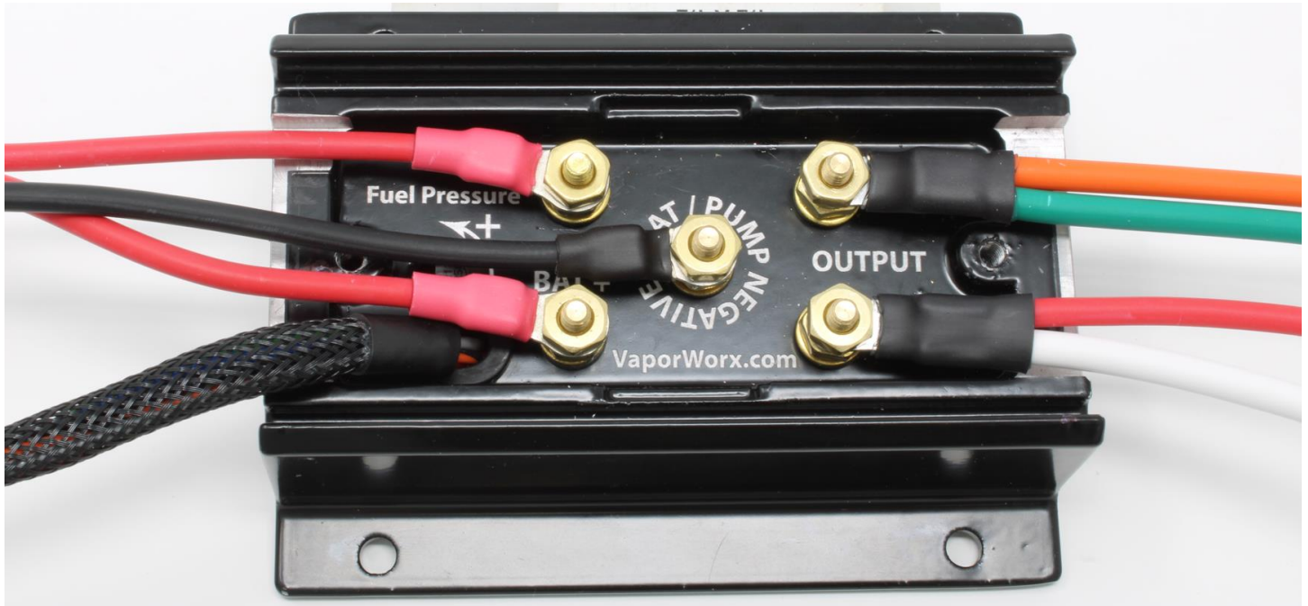
Photo 5. Wiring connections at the PWM Controller.
