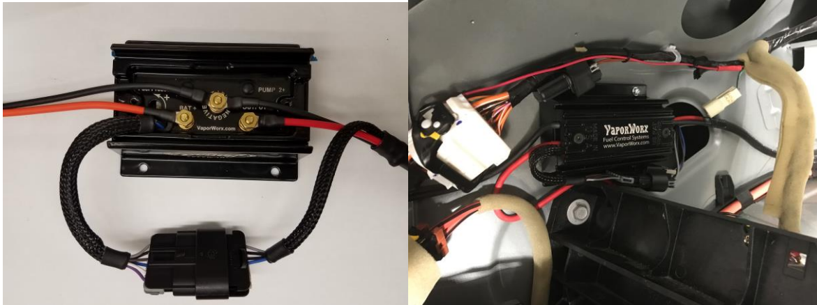
Photos 7 and 8. The wiring from the battery enters from the LH side, to the pump and sensors exits to the right.
